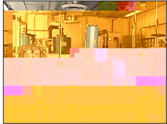
Groundwater treatment center. Source: http://www.tucsonaz.gov/ets/Groundwater/Los_Reales/los_reales.html
